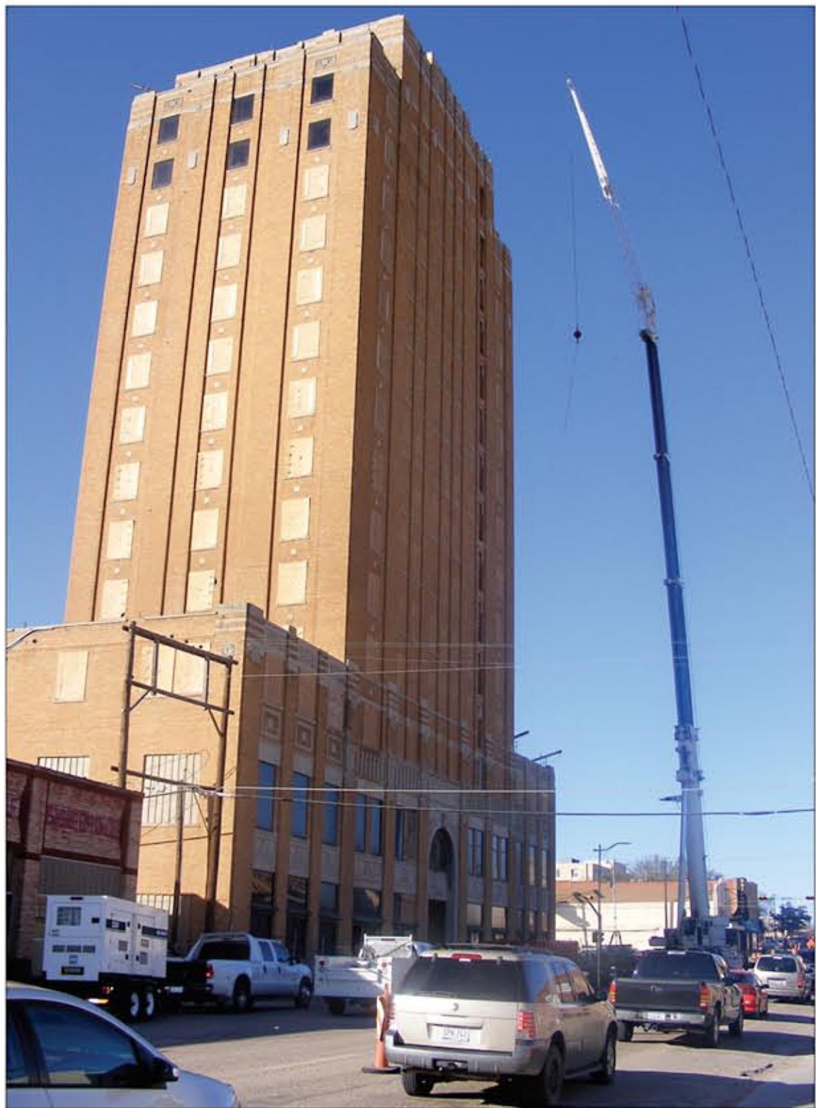
Work crews set up a crane outside the Settles Hotel building this morning. The crane will be used to hoist elevators to the top of the building.
